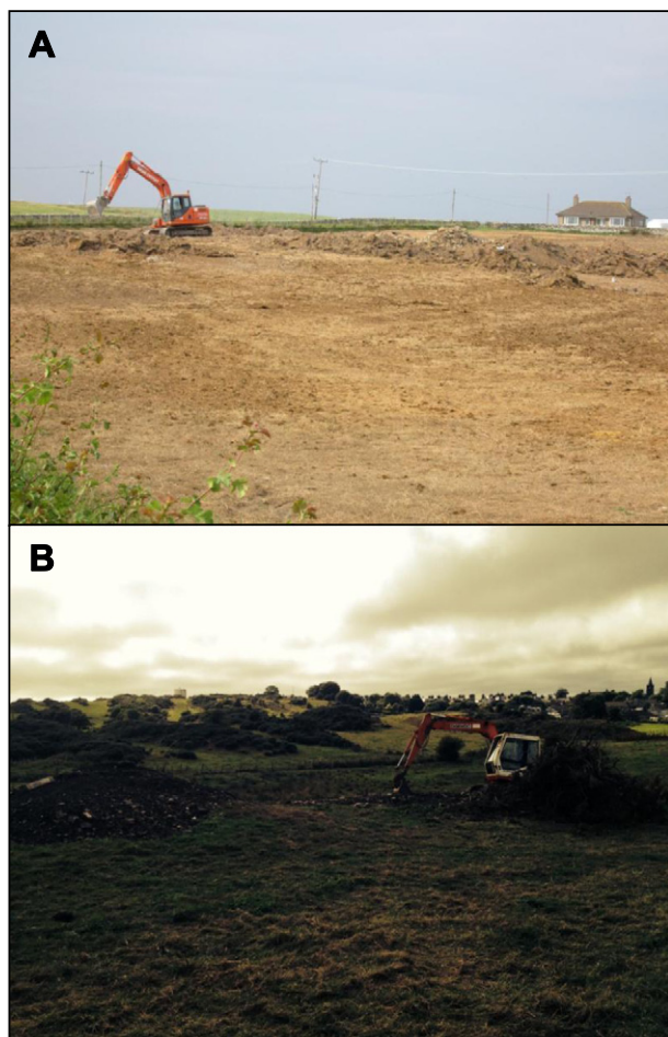
Fig. 9. Man as soil maker: a landscape under change. A) Heavy earthmoving machinery removing the rocky ridges of the Glasserton Rigs and subsequent levelling of the land for agricultural, largely pasture, production. B) Removal of rig features with excavator in foreground with good examples of rig features on display in the background.
